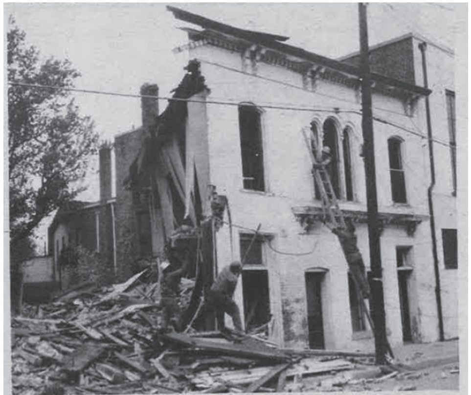
GOING, GOING, GOING. The old Borough Hall on Stockton Street is shown in the process of being torn down in the early 1960's. Since the second half of the 19th century, it housed the Council rooms, the court room, the men and women's jails, the water and sewer office (after water and sewer came to Hightstown), the tax office and the fire equipment until the new firehouse was built in 1928. The land is now owned by Allen and Stults.
